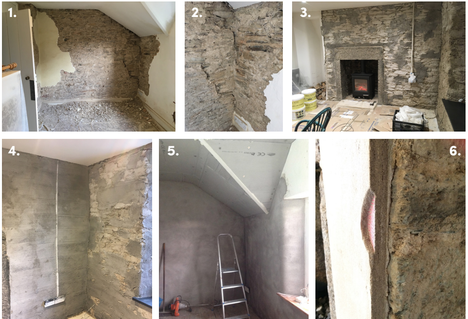
1. Stripping the existing plaster. 2. Repair structural cracks. 3. Harling to key and fill holes. 4. Scratch coat with key. 5. Float coat and final skim finish. 6. End view of layers with mesh.
